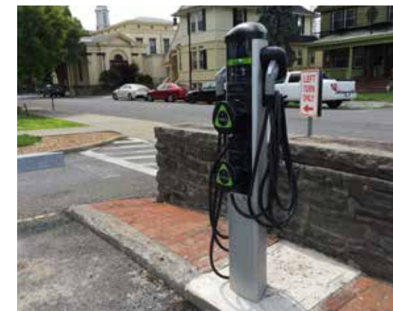
Electric Vehicle Charging Station at the Ulster County Office Building.
