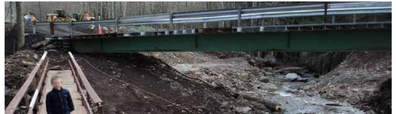
Culvert washout. Ulster County Culvert Assessment Project
