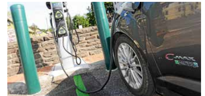
EV Charging station at the Ulster County Office Building. Daily Freeman
