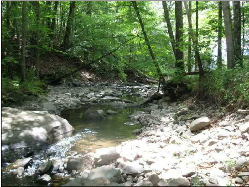
Photo 20. Butternut creek, looking south from failed culvert.
